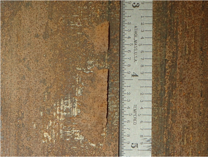
Figure 11. Image of the ID of a wall thickness variation anomaly.
