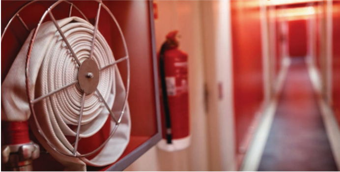
Fire & Safety Systems Inspection
