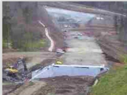
Client: DGF (Spain)
