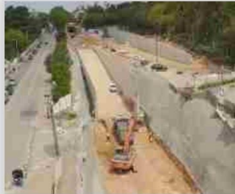
GEOTECHNICAL INSTRUMENTATION AND MONITORING FOR METRO PORTO. YELLOW LINE (PORTUGAL)
