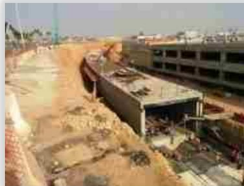
INSTRUMENTATION AND MONITORING OF NORTH LAUNCHING SHAFT 5C2 STATION AND CENTRAL SHAFT. LOT 3 (LINE 5), RIYADH METRO PROJECT
