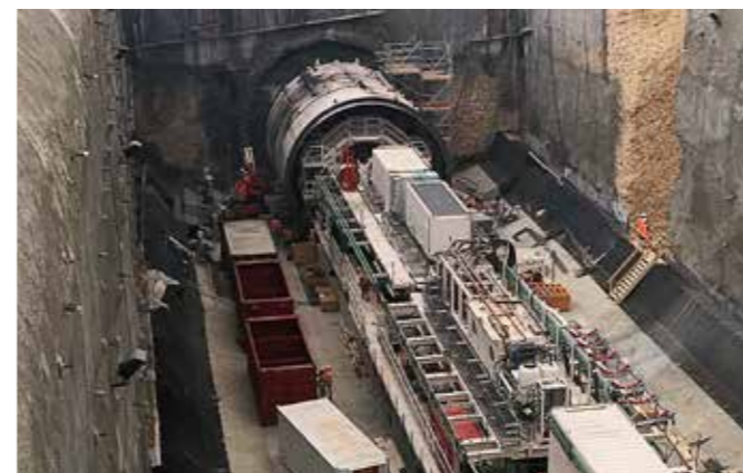
Instrumentation and Monitoring of North and Central Launching Shafts, (Line 5), Riyadh Metro. KSA
