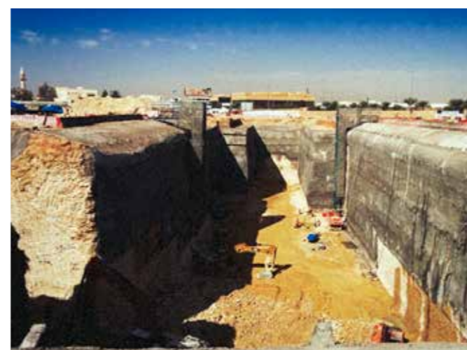
Instrumentation and Monitoring of North and Central Launching Shafts (Line 5). Riyadh metro. KSA.
