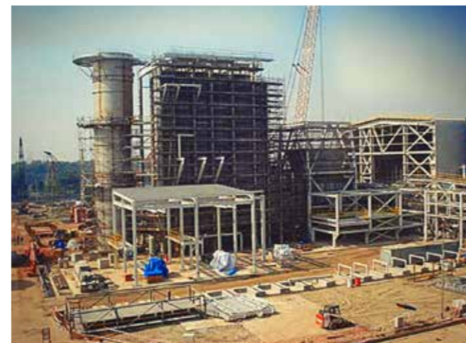
Combined Cycle Power Plant of Asughan (TSK). Bangladesh
